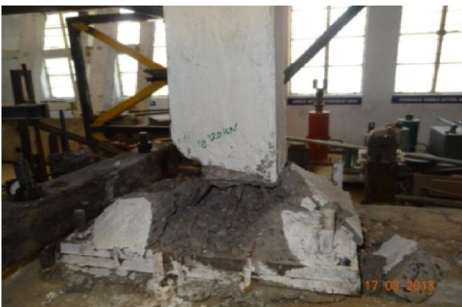
Figure 4. Final failure of frame
