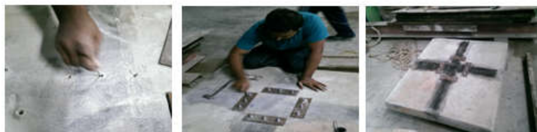
Fig.5. Installation of anchors carried out as per previously specified steps in this project work
