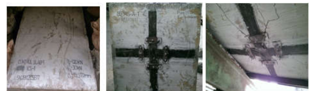
Fig .8. Crack pattern of control slab and retrofitted slab, Mode of failure: Fracture of FRP and Failure of anchor Bolt
