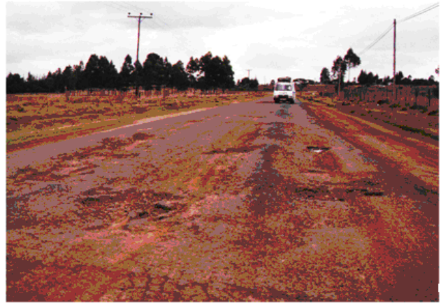
Plate 2: Potholed section of Kesses-Cheptiret Road
