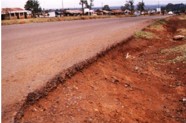
Plate 4. Eroded edge of the road along Kesses – Cheptiret Road at Kesses Centre
