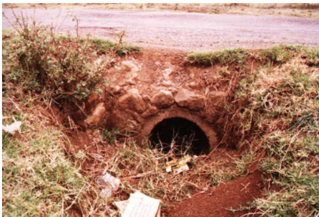
Plate 1. Silted up culvert entrance along Kesses-Cheptiret Road
