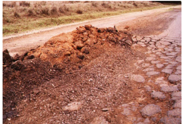
Plate 3: Completely failed road base along Kesses – Cheptiret Road
