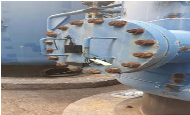
Figure 3. The smart label attached to a tank
