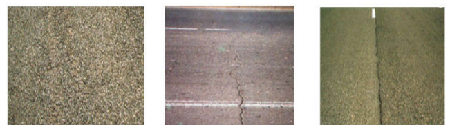
(a) Chunking (b) Transverse cracks (c) Joint crack
