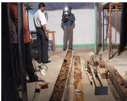
Fig 4. Documentation of Extent of deterioration by termite in beam
