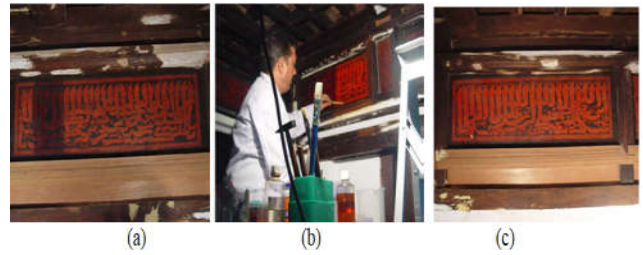
Fig 5. Filling of frame inside the mosque deteriorated by termite- (a) before (b) during and (c) after conservation
