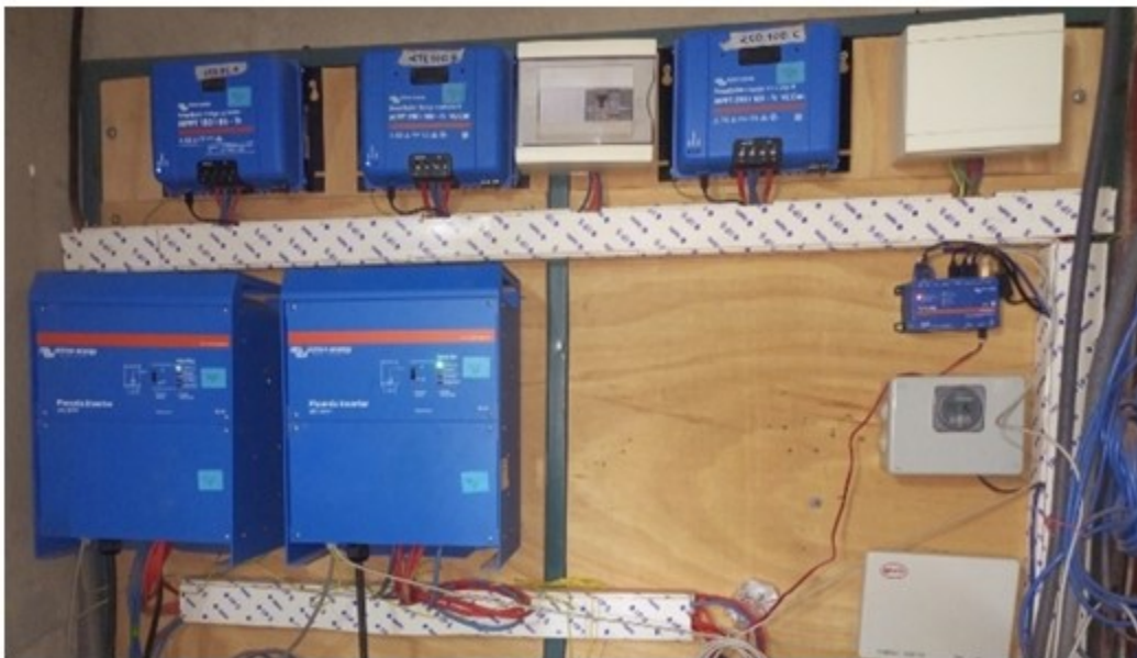
Figure 1. Solar electrical panel of site
