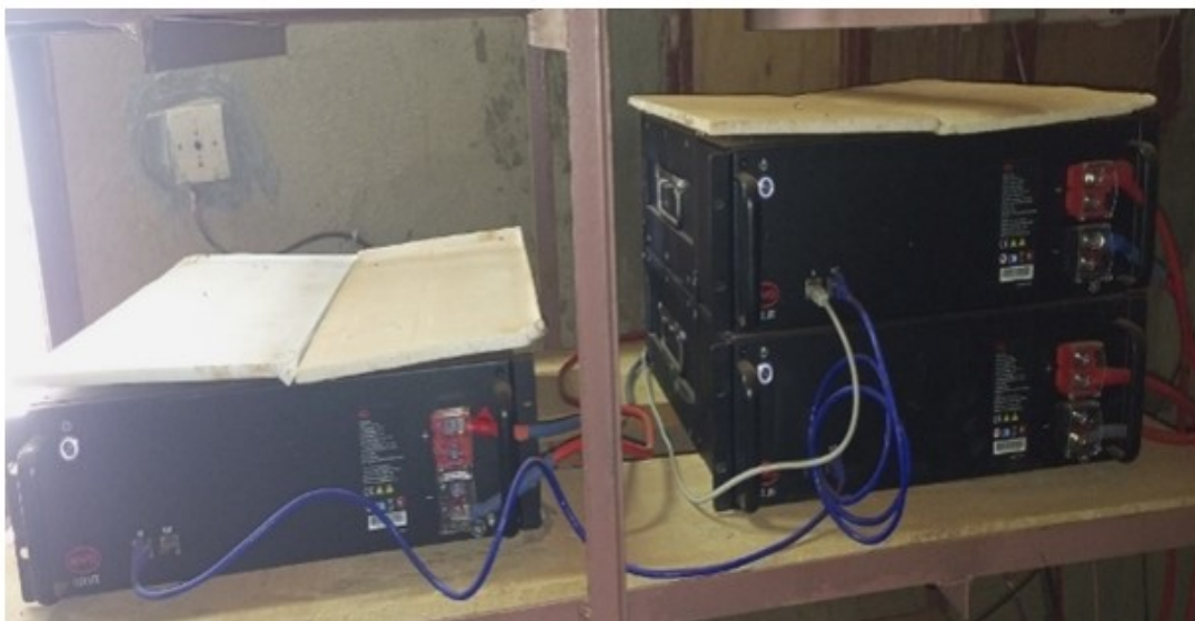
Figure 8. Lithium battery park of site
